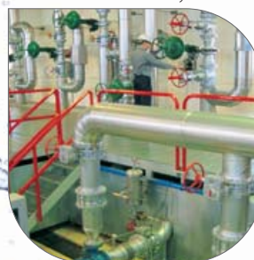
<< Industrial Process Systems
