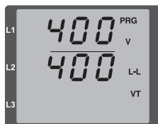
Fig. Programming mode Voltage transformer The primary and secondary currents can be changed using buttons 1 and 2 (cf. page 41).
