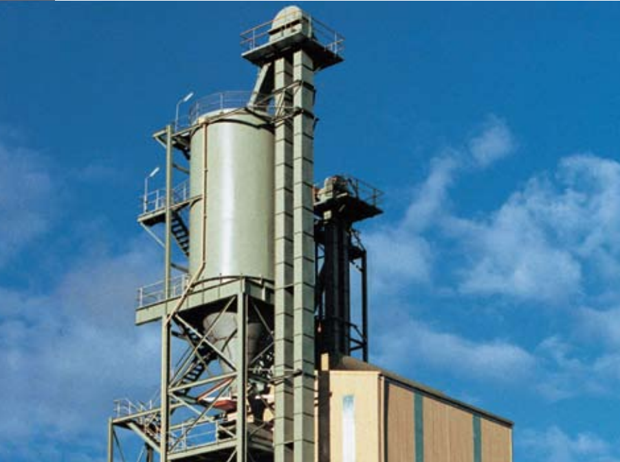
Silo feeding by high performance bucket elevator using central chains.
