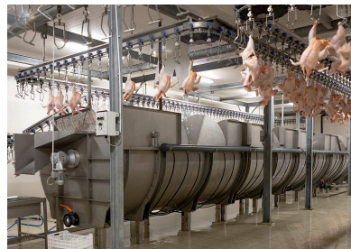
Chilled water Dosage: 30-60 ppm PA
