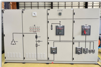
MDB Panel & Enclosure
