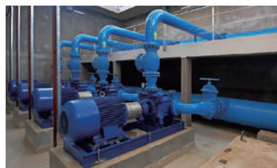
Building water pumps
