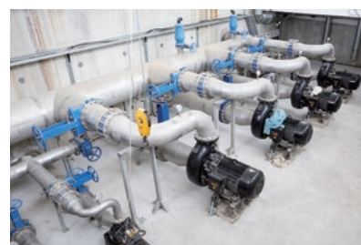
Sewage treatment plant
