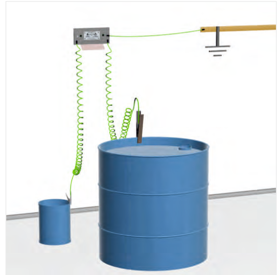
To remove static electricity from the EX/HAZLOC atmosphere grounding clamps should be capable of achieving connections to equipment with resistance values that do not exceed 10 ohms.
