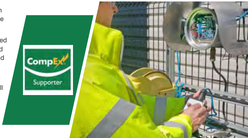
Our CompEx certified engineers commission and service all Newson Gale static grounding and bonding equipment installed at your site.
