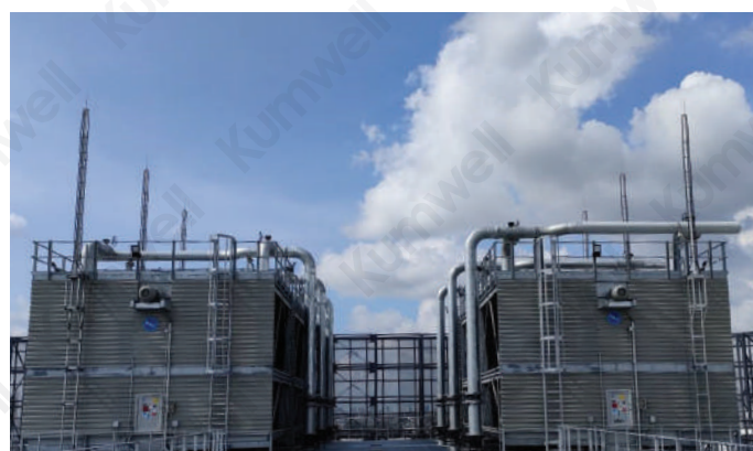
KHV Cable Application on Data Center Rooftop
