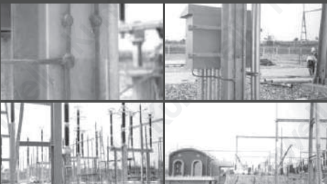
THAILAND : 230/500KV, PLUAK DAENG ELECTRICITY GENERATING AUTHORITY OF THAILAND, (EGAT)
