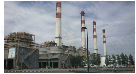
THAILAND : PTT GASSEPARATION PLANT
