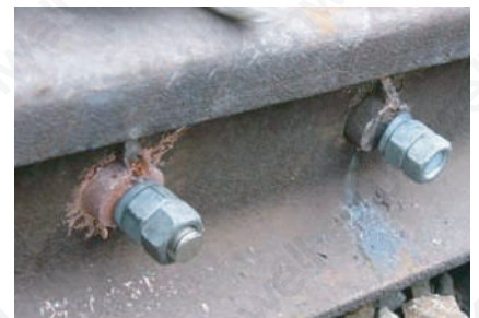
Stud to rail
