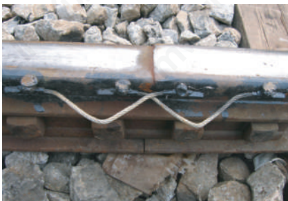
Signaling cable to head rail
