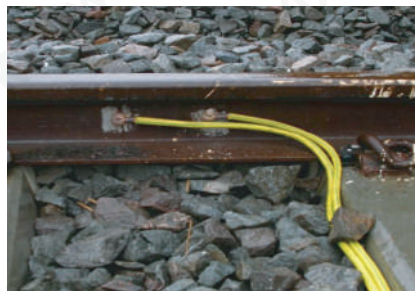
Signaling cable to web rail
