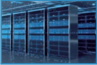
Ohio / Virginia Web Service Data Center 60 MW
