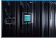
Thailand Telecom Data Center 5.2 MW
