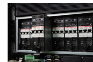
Hot-swappable breaker module
