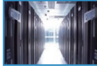
Vietnam HTC-ITC Data Center Uptime Tier III TCCF 750 kW
