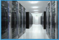
Washington Data Center 17 MW
