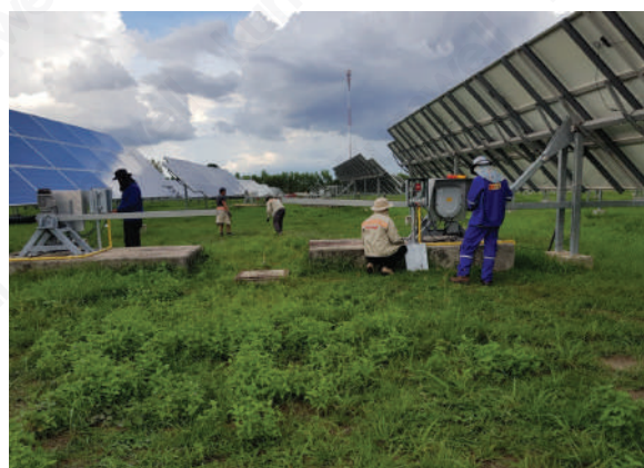
THAILAND : Solar Farm EGCO SPPS (Roi-Et)
