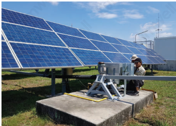
THAILAND : EGCO Solar Farm
