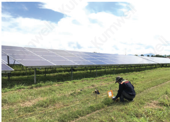
THAILAND : Super Energy Solar Farm
