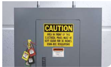
Panel & Enclosure ID
