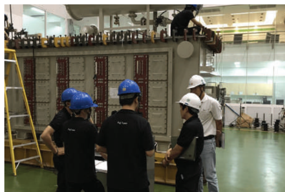
Transformer inspection and testing
