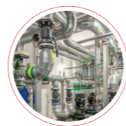
Fan and Water pump
