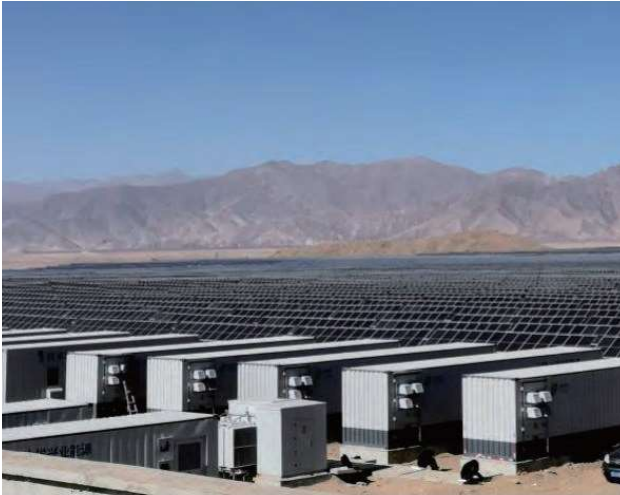
○ Tibet Light Storage Comprehensive Energy Project
