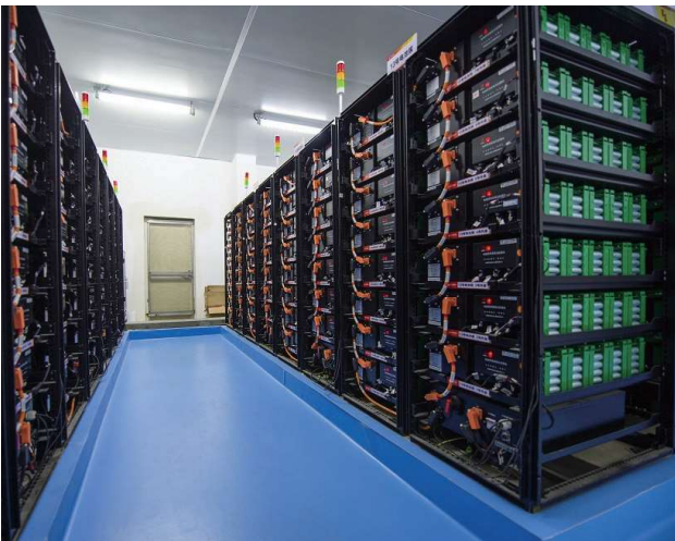
○ Kunshan Industrial Park Energy Storage Project
