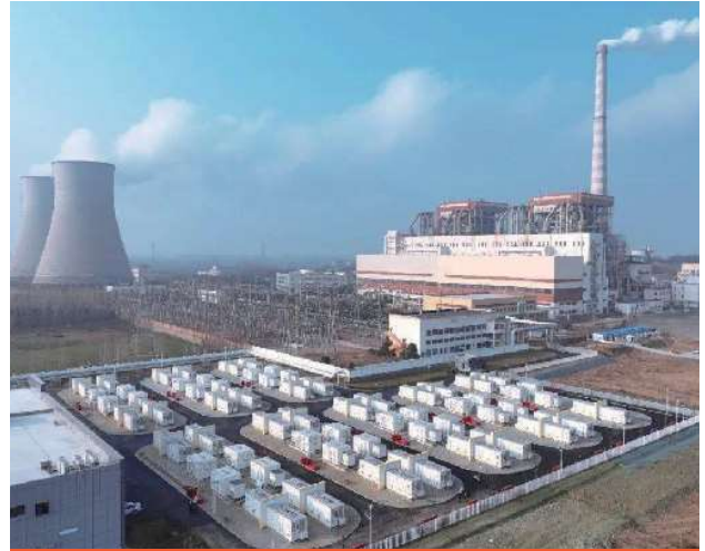
○ Huaibei Wanneng Energy Storage Power Station Project
