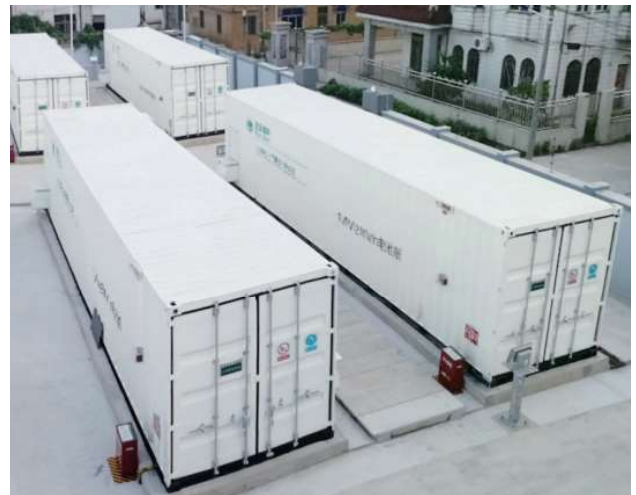
○ State Grid Zhenjiang Changwang Energy Storage Project
