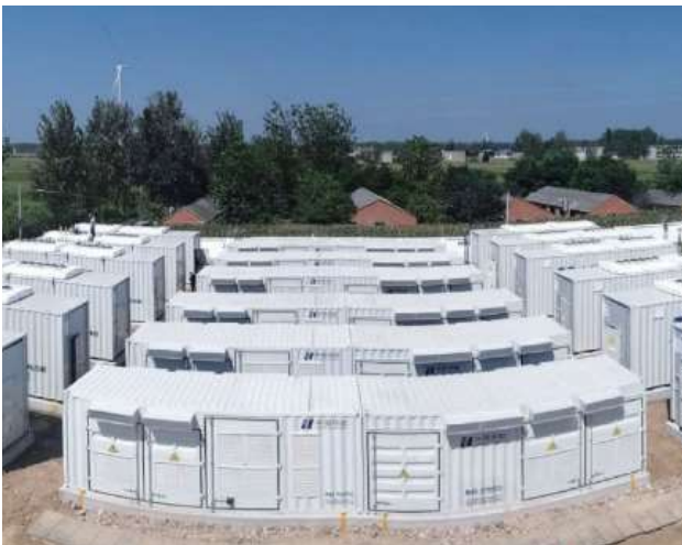
○ Huaneng Wind Energy Storage Frequency Modulation Project
