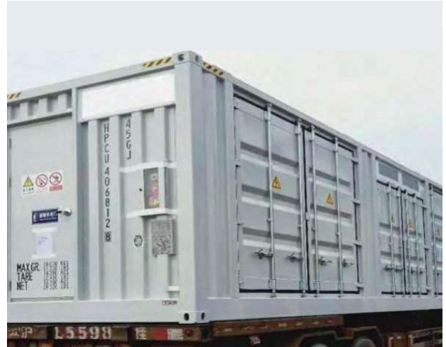
○ Dubai Light Diesel Storage Microgrid Project
