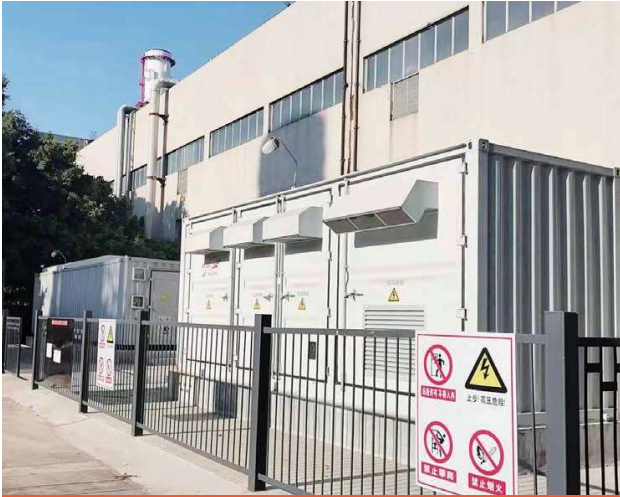
○ Shenzhen Nanshan Power Plant Frequency Modulation Project
