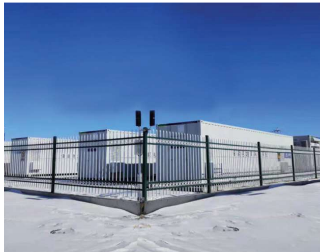
◎ Shangneng Zhangjiakou Solar Energy Storage Project
