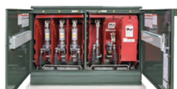
15b. PMH Pad-Mounted Gear (Communicates when Remote Supervisory)
