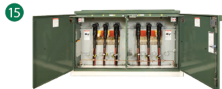
15a. PME Pad-Mounted Gear (Communicates when Remote Supervisory)
