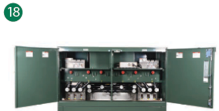
18. Vista ® SD Underground Distribution Switchgear PMH or PME Configuration (Communicates when Remote Supervisory)
