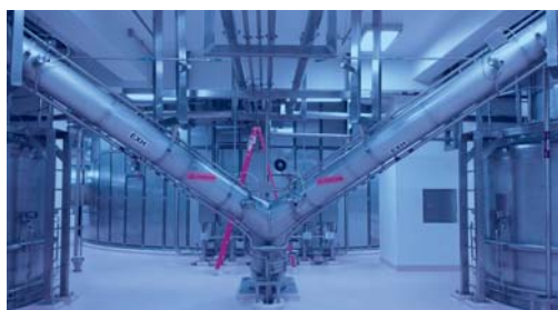
DRYER EXHAUST DUCT & CIP LOOP
