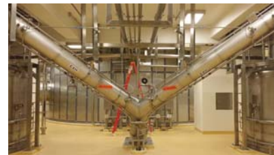
DRYER EXHAUST DUCT & CIP LOOP
