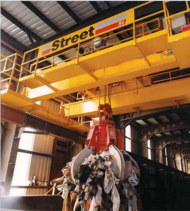
Waste to energy application control room operation or full automation
