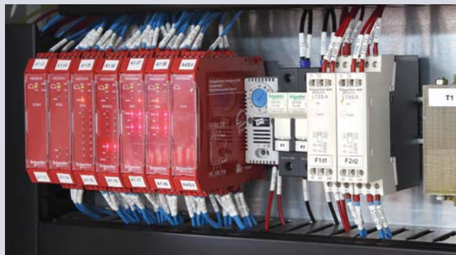
Category 3 safety rated controls
