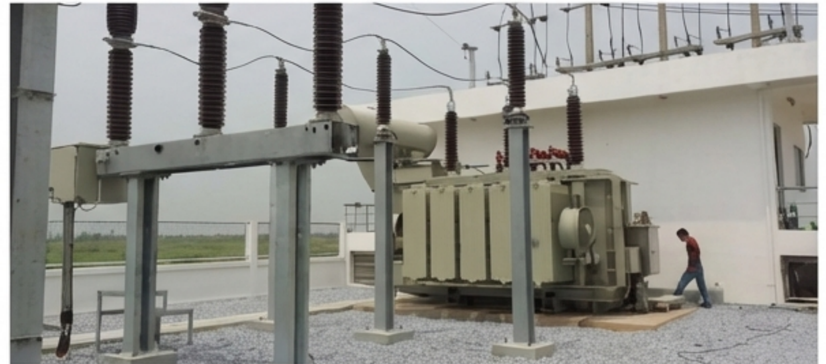
115kV Substation - Cargill Korat
