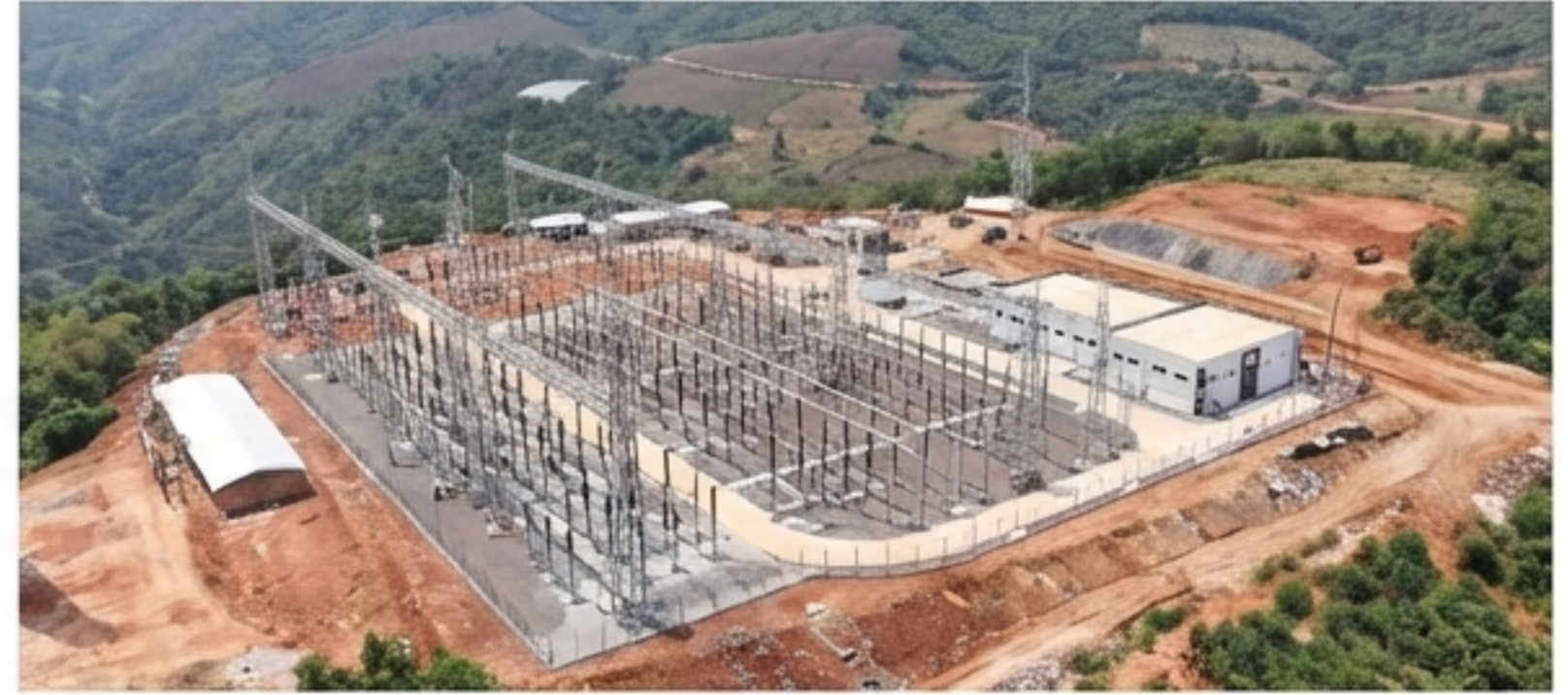
220kV Switching Station - Nam Emoun, Laos
