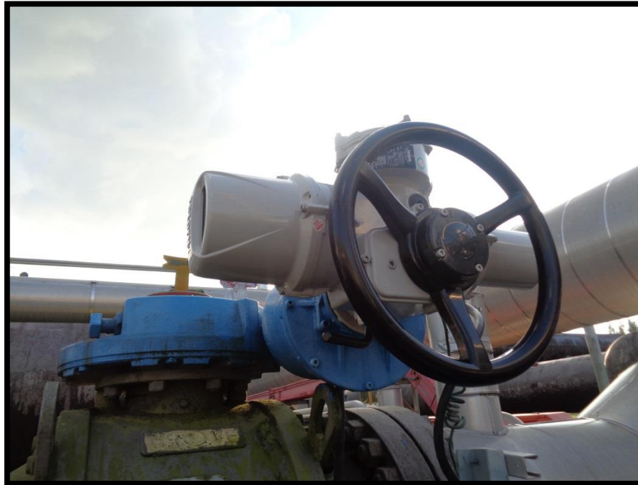
Installation Actuator at Site
