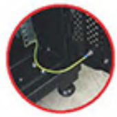
Grounding System Connecting Between all Removable Part of Rack with Copper Ground Wire 2.5mm 2
