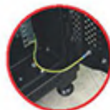
Grounding System Connecting Between all Removable Part of Rack with Copper Ground Wire 2.5mm 2
