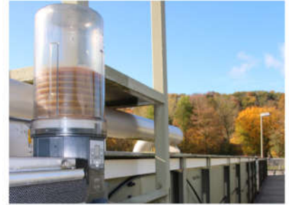
Industry: Sewage treatment plants Application: Rotary screen
