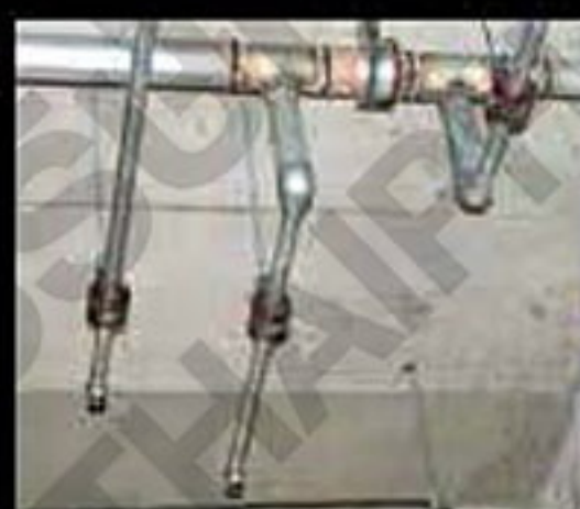
Fire Sprinkler Systems
