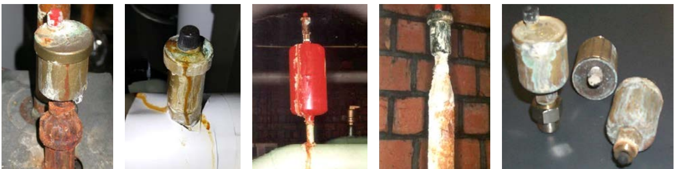
Example of poor-quality air vents, which soon begin to leak due to their faulty construction
