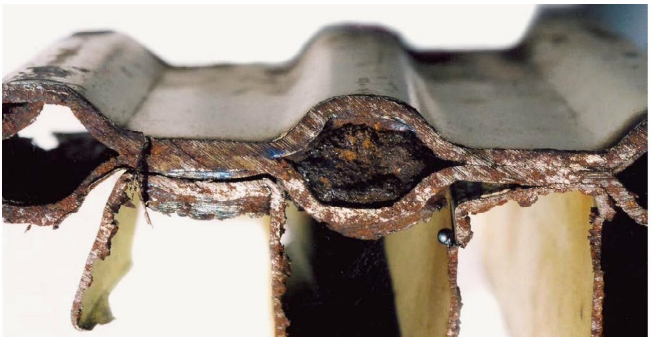
Typical consequences from poor water quality management.
