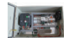
Crane Cabin and Control Panel 91-96 NTC Control Cabin NCP Long Travel Control Panel
