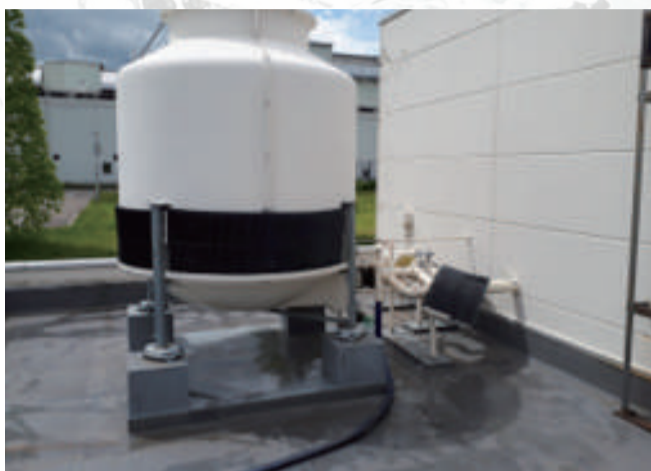
▶ Cooling tower water treatment
