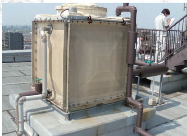
▶ Elevated tank water treatment
