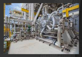
Oil & Gas Equipment
