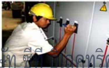
CIRCUIT BREAKER INSPECTION
