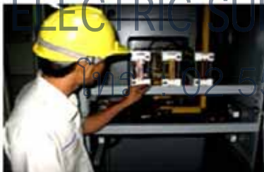
BUSBAR SUPPORT INSPECTION
