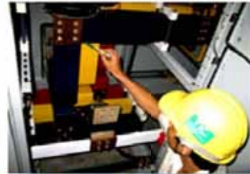
COPPER BUSBAR INSPECTION NUT, BOLT, SCREW
