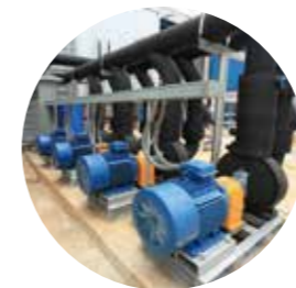
Area pump control
