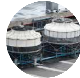
Cooling tower energy saving
