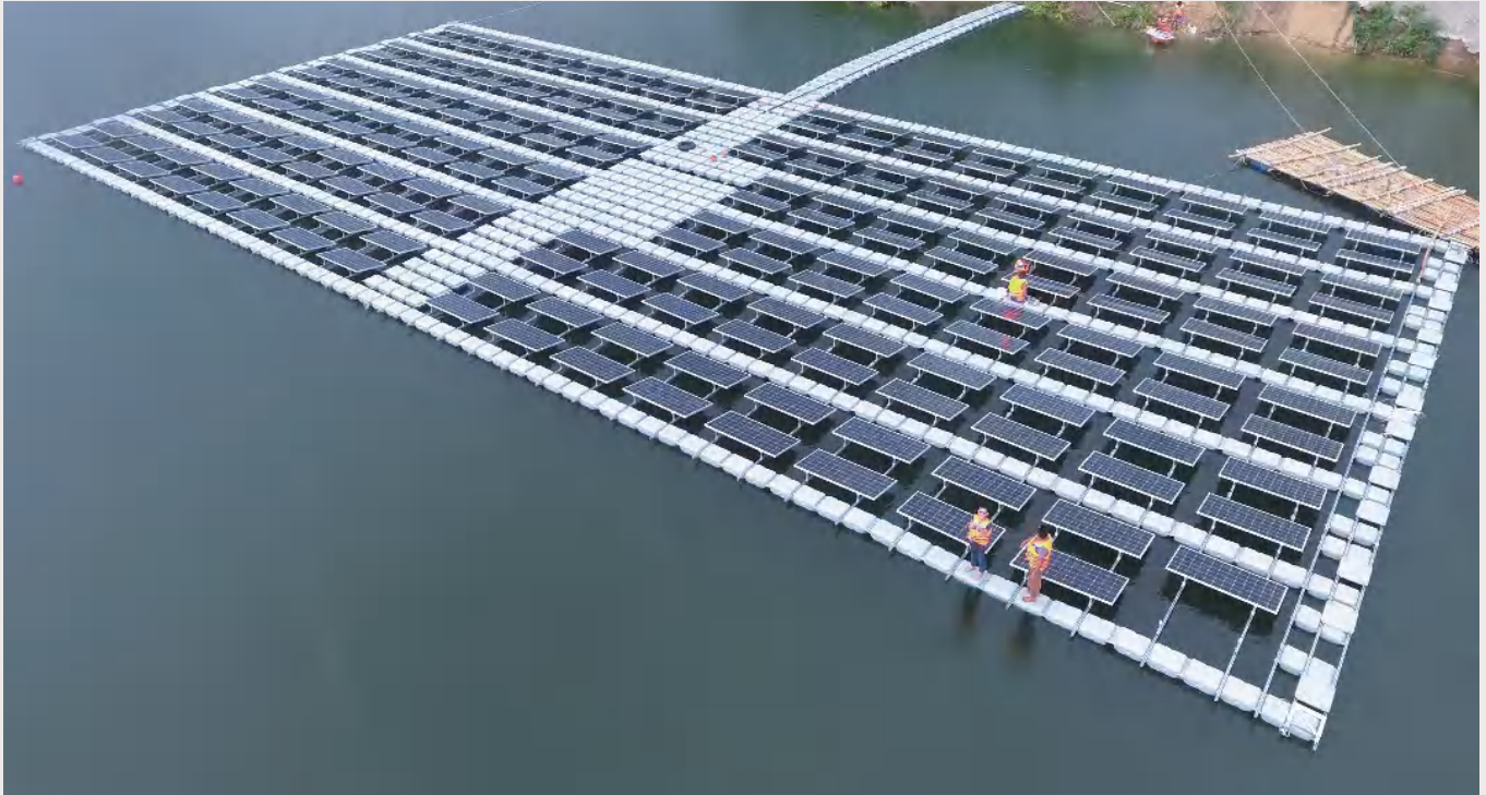
INDONESIA 100KW FLOATING PHOTOVOLTAIC POWER PROJECT
