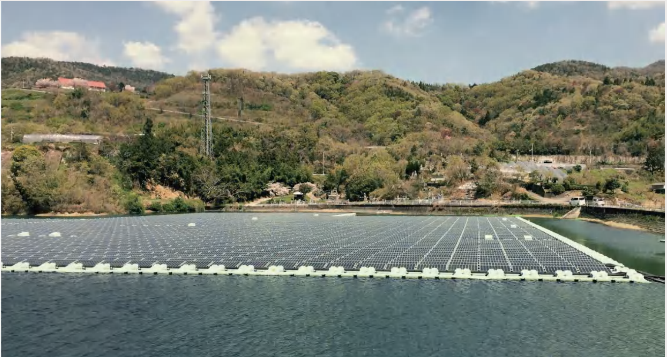
JAPAN 5MW FLOATING PHOTOVOLTAIC POWER PROJECT
