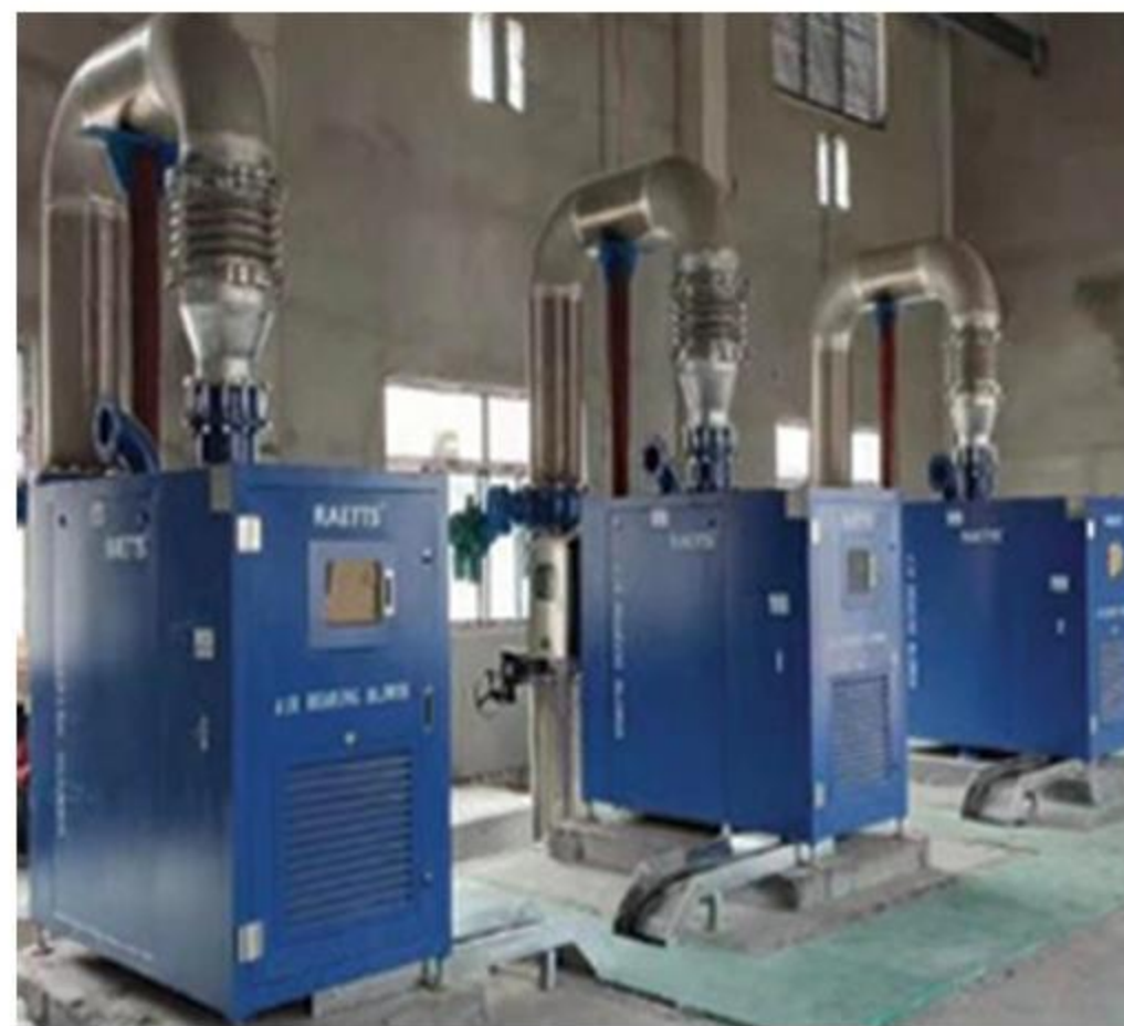
Sewage treatment factory in Yicheng County, Linfen
