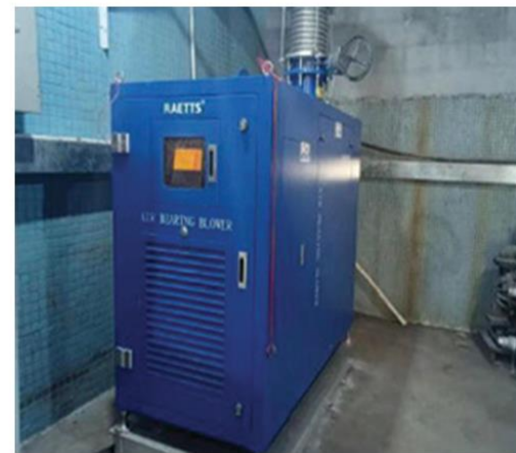
Sewage treatment factory in Dongguan
