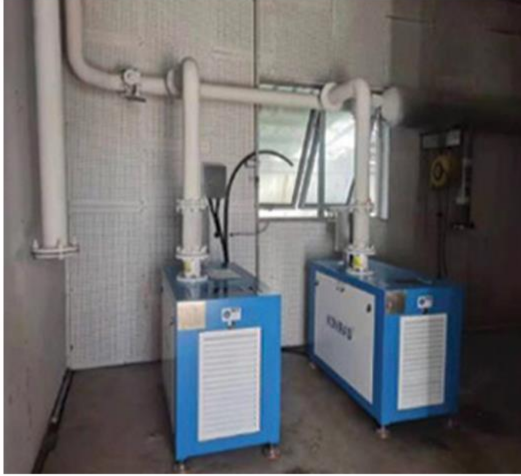
Sewage Treatment Station In Xuzhou Tongshan District
