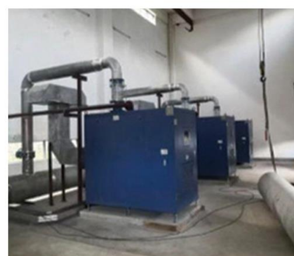
Sewage treatment factory in Lincang County, Yunnan
