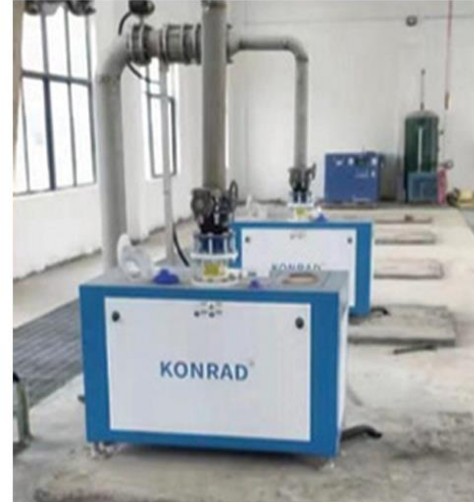
Sewage Treatment Station In Xuzhou Tongshan District
