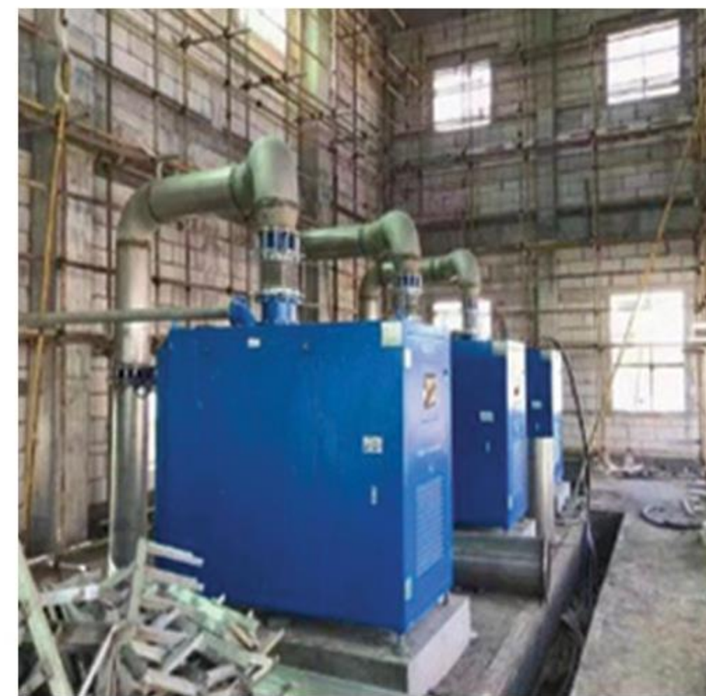
50,000 tons of sewage treatment in Anhui
