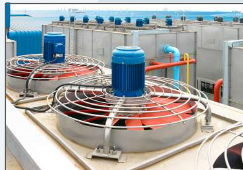
Fans and water pumps
