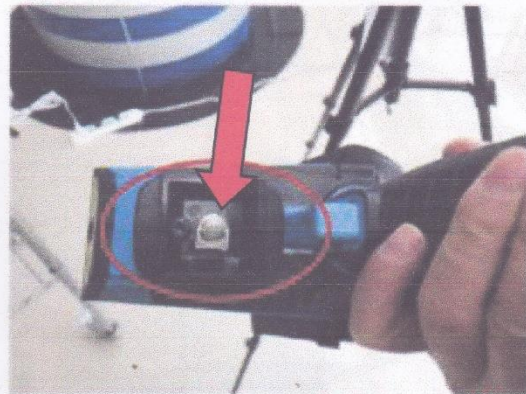
2, Wrong horizontal installation
