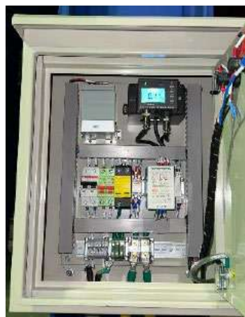
Smart Ground Monitoring
