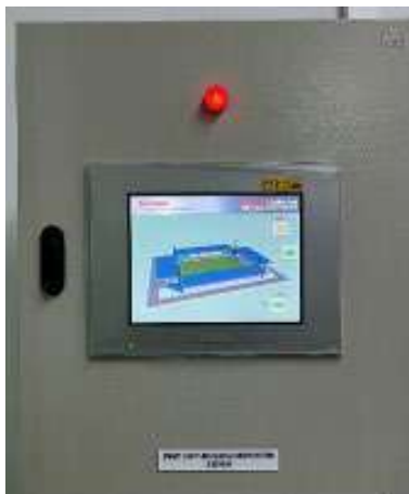
Smart Lightning Management System
